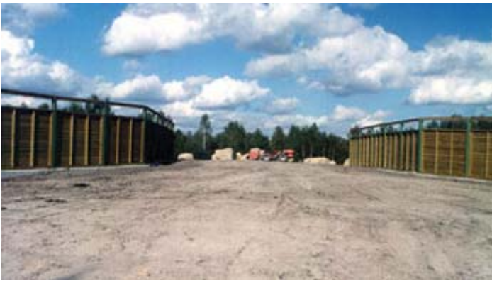
A French 'hour glass' example with solid screens for fencing, as viewed from the fauna approach side
